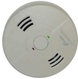
Smoke & CO Detector
